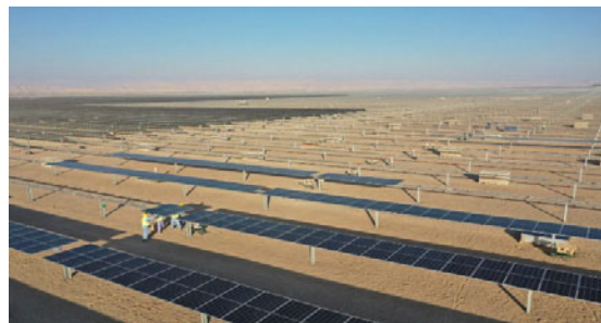
Workers installing one of 1.4 million solar panels that make up the Ibri II 500-megawatt solar photovoltaic independent solar power plant, the largest utility-scale solar park in Oman. Photo © AIIB 2021
