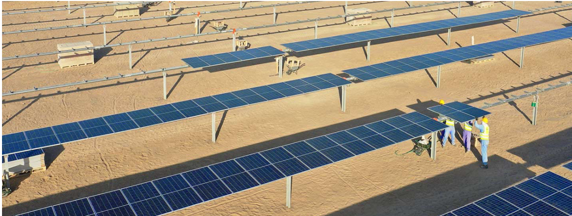
Workers installing one of 1.4 million solar panels that make up the Ibri II 500-megawatt solar photovoltaic independent solar power plant, the largest utility-scale solar park in Oman. Photo © AIIB 2021
