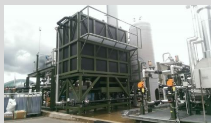
Biogas upgrading plant by Frames (© Frames Renewable Energy Solutions)
