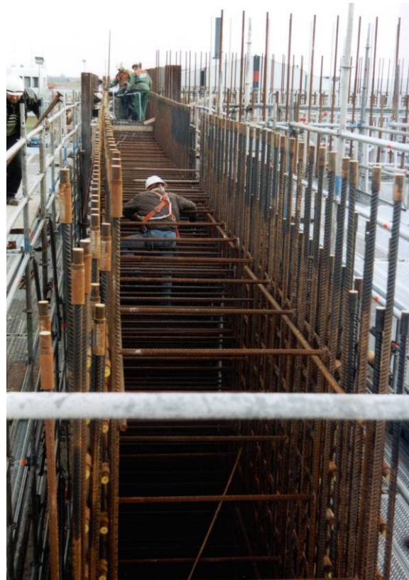
Figure A.5. Worker in the concrete at work in a 1,7 meter thick outer wall
