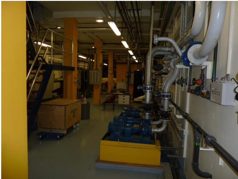
Figure 7-3: Water treatment room in the basement
