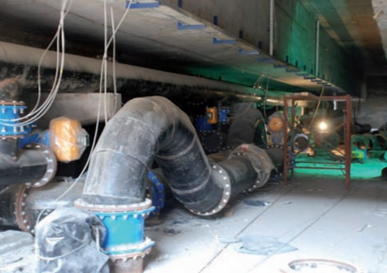
Filter house New El Azab Water Treatment Plant
