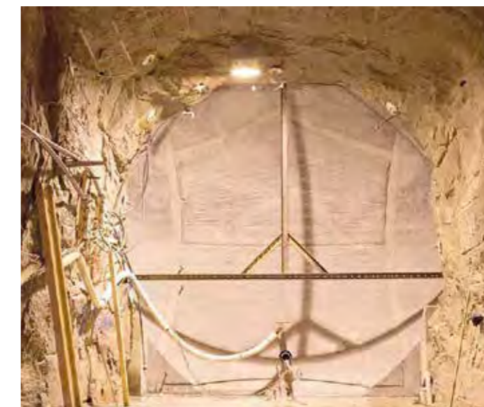
Figure 2-7: The cast concrete face of the composite DOMPLU test disposal tunnel plug at the Äspö URL in Sweden (image: SKB).
