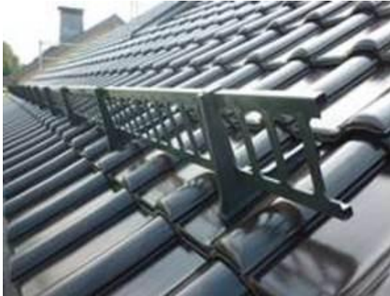
Figure 30 Snow guard rails to capture loose tiles.
