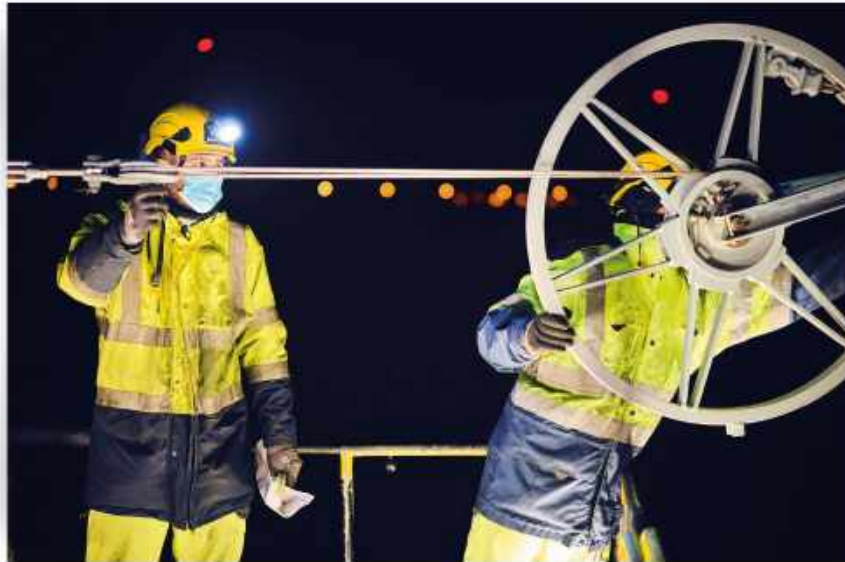
Electrification works on the line between Mol and Hamont Photo: Infrabel – Benjamin Brolet
