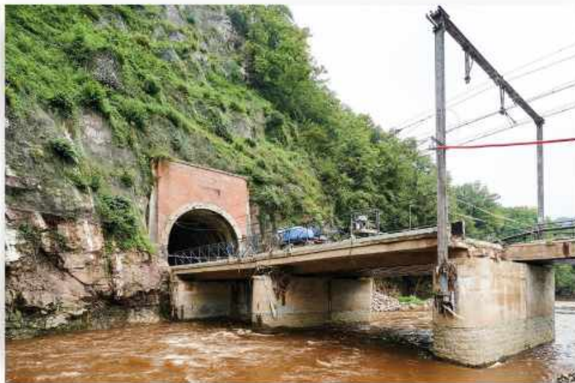
Damaged bridge during the floods in Belgium in July 2021 Photo: Infrabel – Benjamin Brolet
