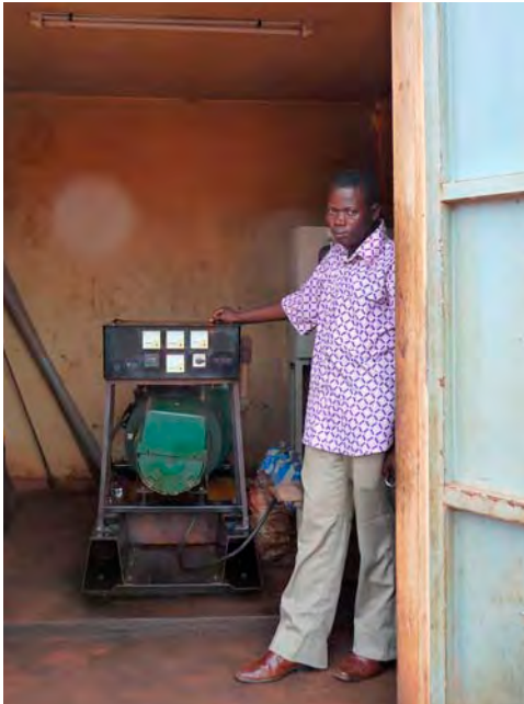
Exploitant small piped water supply system
